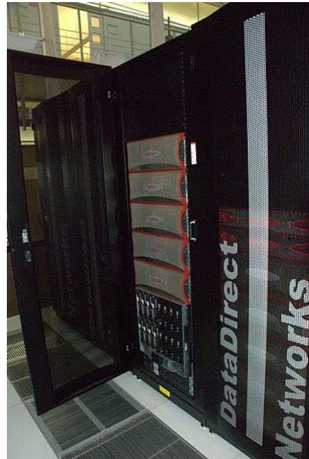
Fig. 13 View of the 1 PB disk storage array installed at PIC in 2009 where the data of the Tier2 is located.
